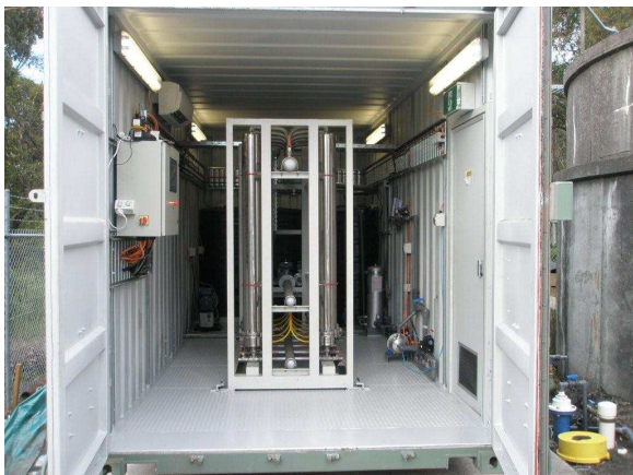
Containerised VPMF Potable Water Treatment Plant
